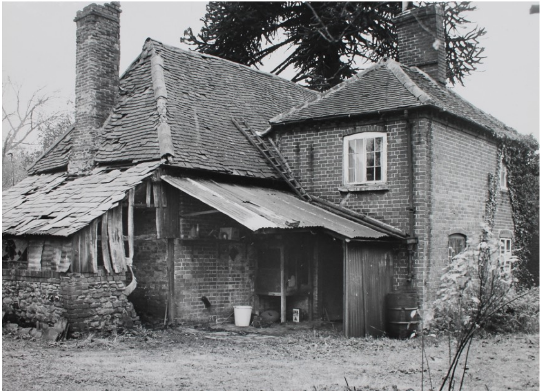
These two images from 1969 show just how dilapidated the property had become.
